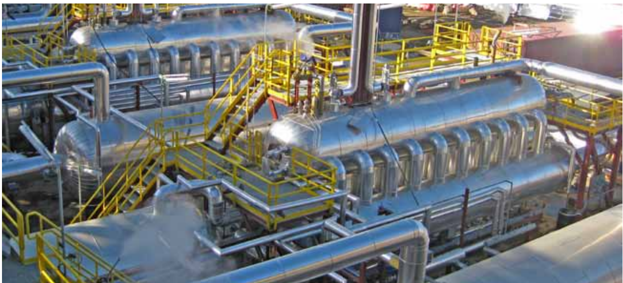
Fig. 1: 50MWe steam generator system for parabolic trough CSP power plant
